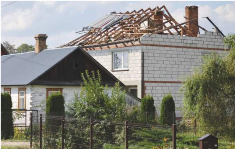
A destroyed roof of a house, after Russian drones violated Polish airspace, in Wryki near Lublin, Poland, Wednesday.
